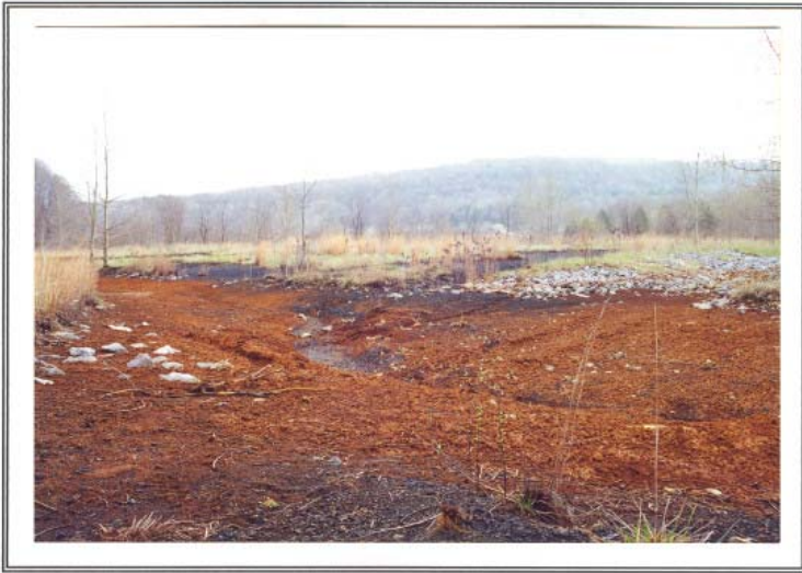
Exhibit 2.4 (J) Looking southwest towards town from the Yellow Boy Channel. To the right will be the wetlands, to the left of the channel will be the clarification marsh. Notice the patches of boney and some rip rap.
